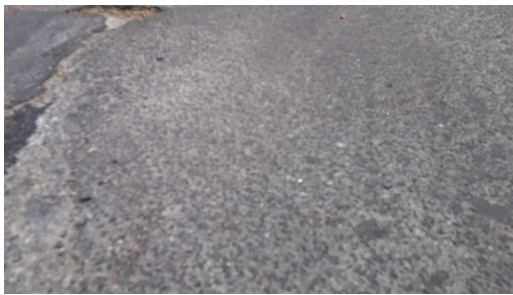
Fig. 16. Image of a pothole lies in the top left corner
