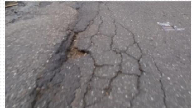
This image is classified as 'Cracks'
